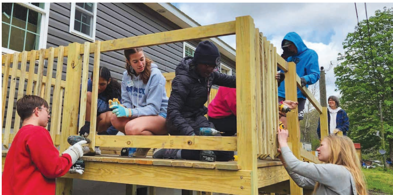
Eastern Mennonite School students build a porch in April on a house constructed by Mennonite Disaster Service in Hurley, Va., following flooding and mudslides that destroyed 60 homes and damaged 200 others in 2021. PHOTO: EASTERN MENNONITE SCHOOL
